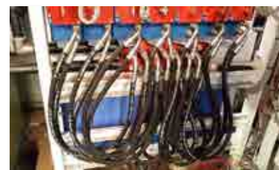
Modules are liquid-cooled using cooling hoses and manifolds.
