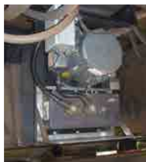
Baltimore Metro blower
