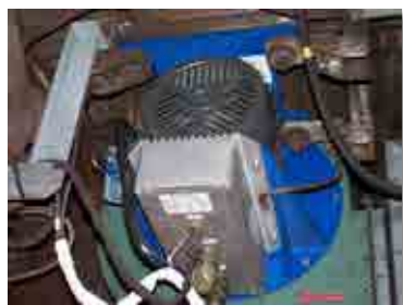
Example of Mini-VFD attached to blower motor
